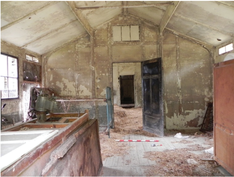
Figure 4. Condition of the treatment wing before the cleaning process began. May 2021. Source: Ana Pastor.
