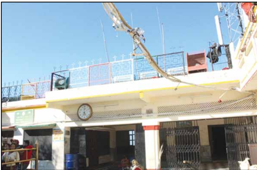
Figure 4: The exposed wiring and lack of maintenance in the temple.
